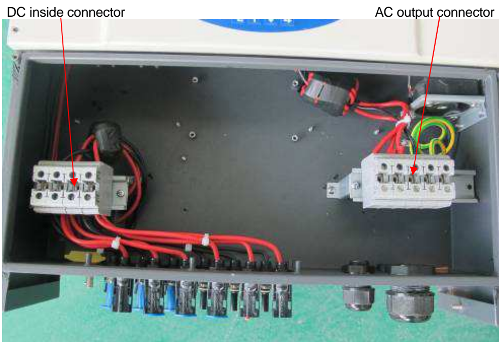
Internal view of the unit
